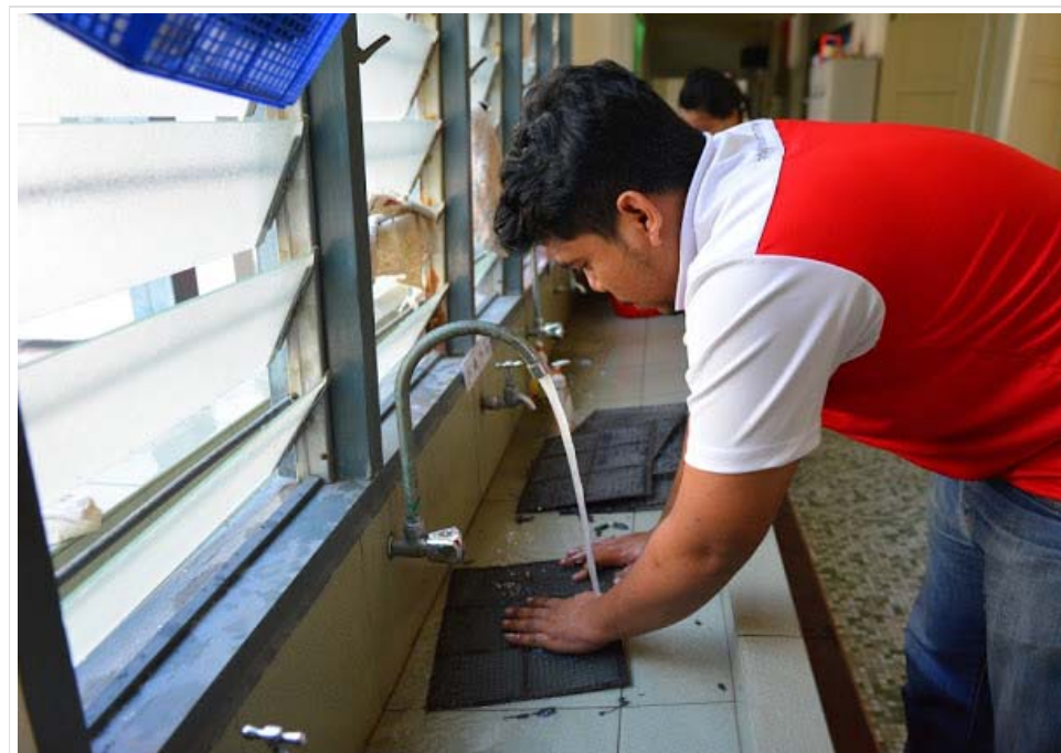
One of the Maintenance associates, Muhamad Azrie, is washing away the dust accumulated on the air-conditioner filters.
